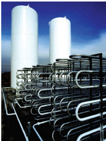
Cryogenic Storage facilities need to be maintained at temperatures as low as -273°C.
